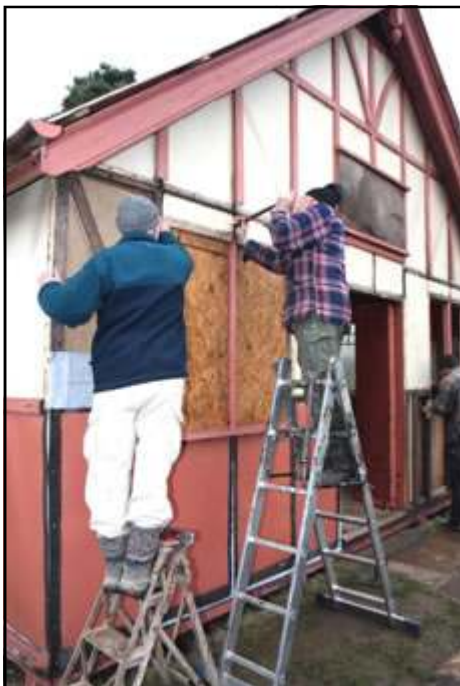
Museum volunteers Ted Beeson and Tom Crosby carrying out repairs on Thame Vicarage Room
